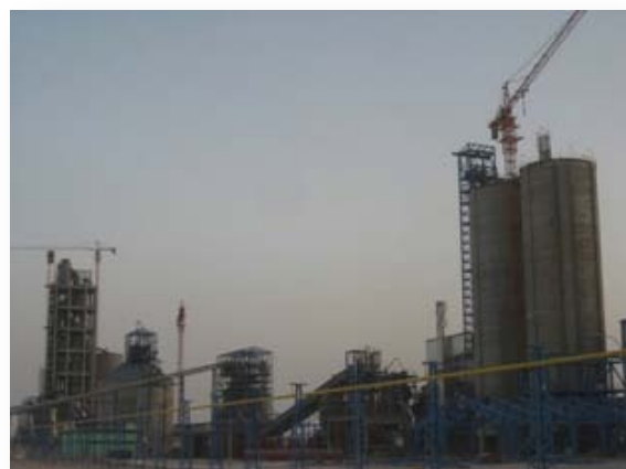
PLANT GENERAL View
