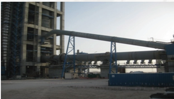
KILN + Pre heater
